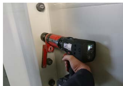
Bolting of vertical flange in the tower with sensor-controlled battery torque wrench MAD 7-S.
